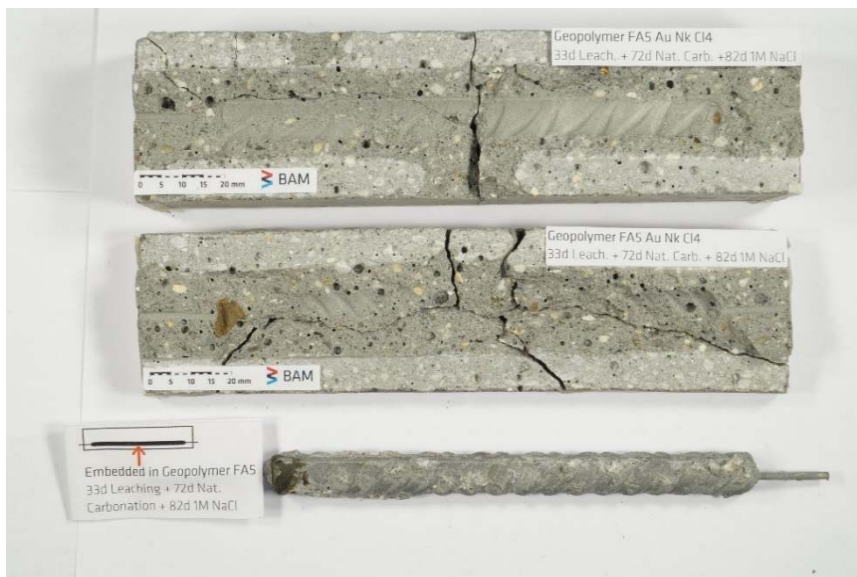
Figure S20. Mortar specimen FA-L-A-Cl 4 and embedded steel rebar split after depassivation of the steel was detected.
