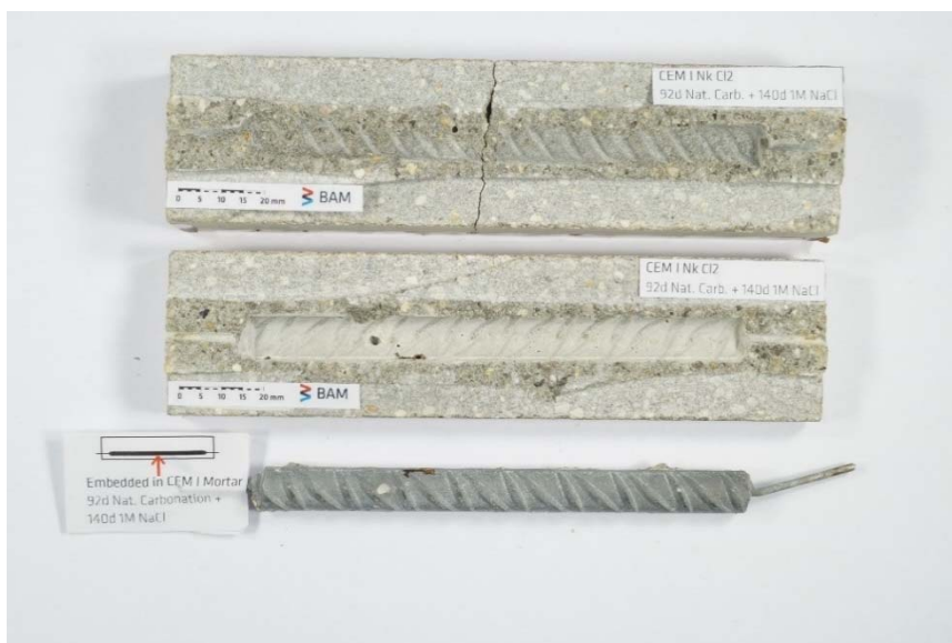
Figure S24. Mortar specimen CEM-CI 2 and embedded steel rebar split after depassivation of the steel was detected.
