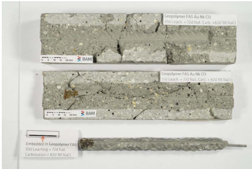
Figure S19. Mortar specimen FA-L-A-Cl 3 and embedded steel rebar split after depassivation of the steel was detected.
