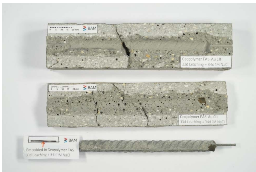
Figure S12. Mortar specimen FA-L-Cl 1 and embedded steel rebar split after depassivation of the steel was detected.
