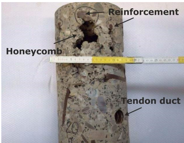
Fig. 6. Drilling core from real structure with honeycomb/ void under reinforcement bars
