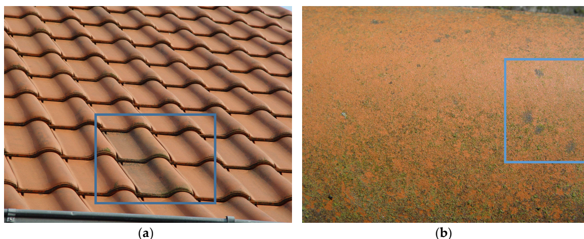
Figure 1. The roof of a residential house with indicated sampled tiles at the moment of sampling in May 2014—after 7.5 years of total exposure and 59 months of exposure beside each other. This area is free from shading by architectural elements and thus photocatalytic activity might occur at least during sun irradiation periods. (a) The position of the two sampled photocatalytically active tiles on the control part of the roof was “home” to those tiles for almost five years prior to the sampling. The photocatalytically active tiles have the visibly different subaerial biofilm that is more discoloring. (b) Sampled tile surface in a close-up showing dark-pigmented fungal colonies on the elevated surface area—the area where time of wetness is additionally reduced, leading to less pronounced algal growth. Fungal colonies that were sampled with sterile implements to isolate dominant subaerial settlers are indicated by the blue frame.
