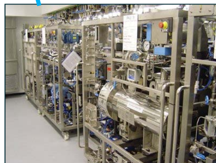
Modular Production (Example: Foster Wheeler AG, Zug/CH)
