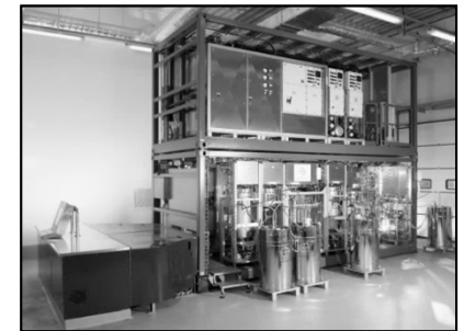
Containerized modular plant Source: INVITE GmbH
