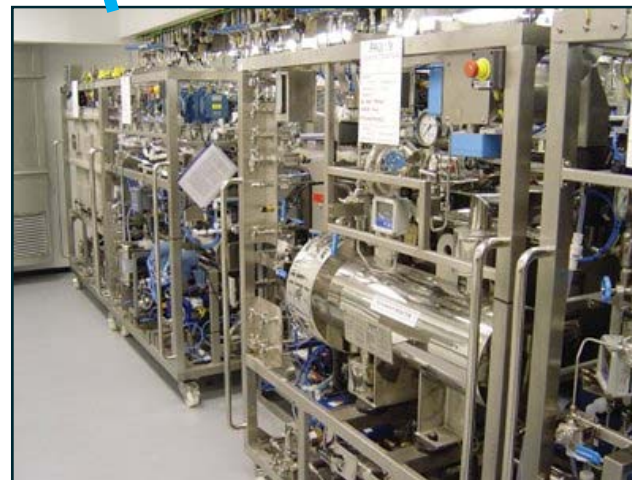
Modular Production (Example: Foster Wheeler AG, Zug/CH)
