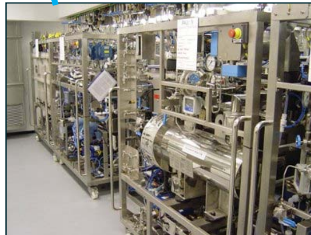
Modular Production (Example: Foster Wheeler AG, Zug/CH)
