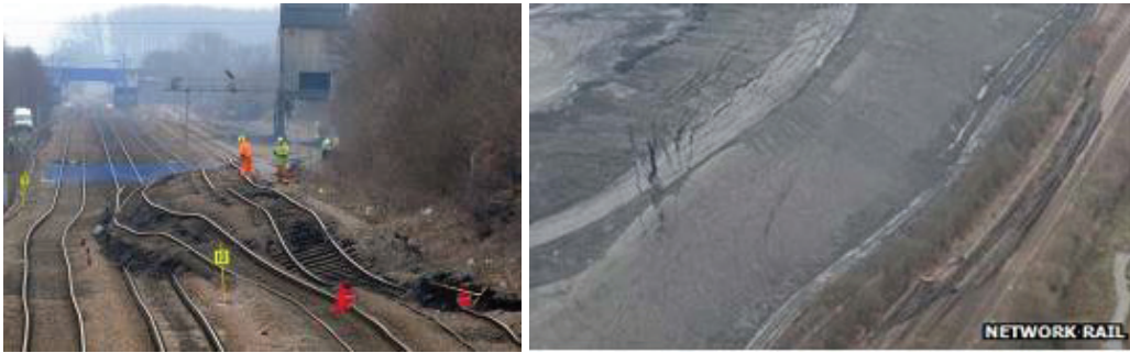
Fig. 2. Landslip rail line in UK, February 2013: view of the railway (left); top view of the area (right).
