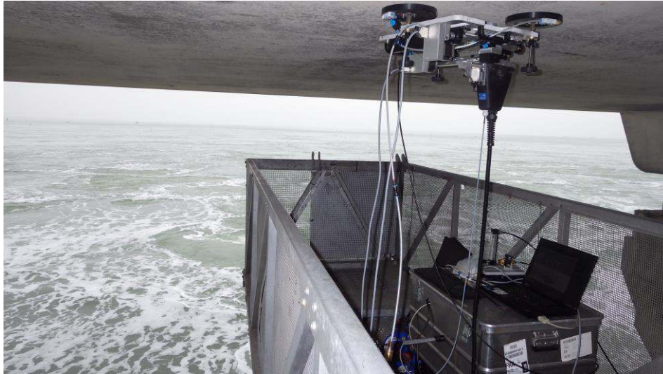
Figure 2. On-site investigation on a bridge; the scanner with the laser-head is fixed with compressed air at the bottom of the bridge to estimate the chlorine concentration.
