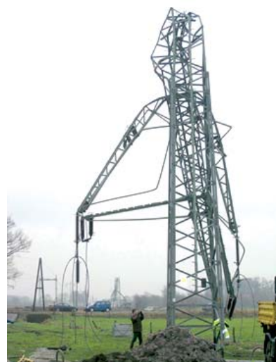
Fig. 8 Collapsed power line transmission tower, due to weather induced mechanical overload
