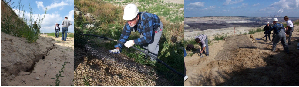
Figure 13. Installation of a geogrid containing PMMA POF at a creeping slope in a brown coal pit near Belchatow, Poland.
