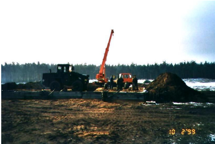
Fig 5.5: The tanking is closed; the remaining gravel is introduced via a ramp using a wheeled loader.
