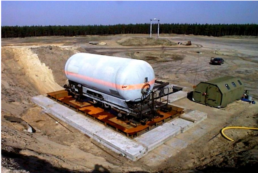
Fig. 3.1: View of the fire stand under construction; the drop tower is seen at the back
